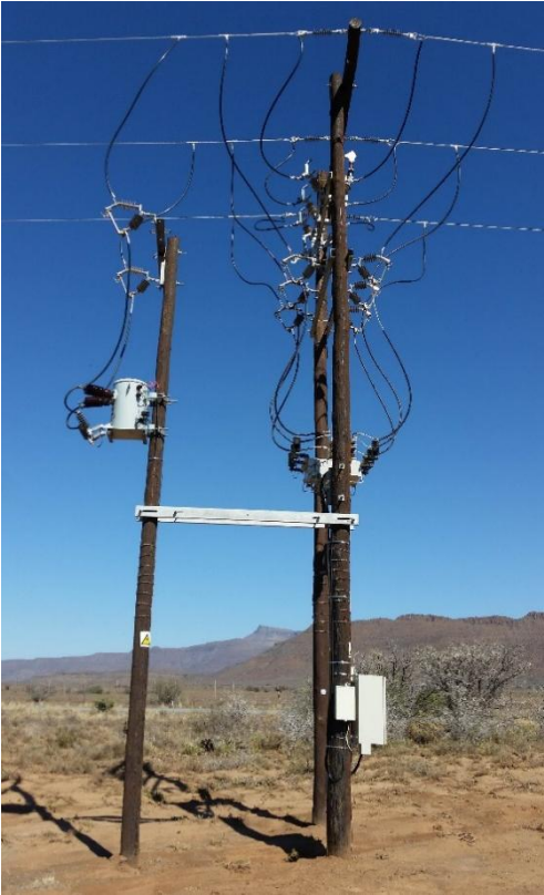
Figure 18: Example of a complex structure with covered jumpers
